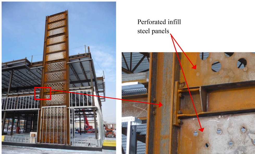
Fig. 2. Four-story perforated steel plate shear wall with RBS-End plate beam-to-column connections (Courtesy of Eric Lachapelle, LAINCO Inc.).
